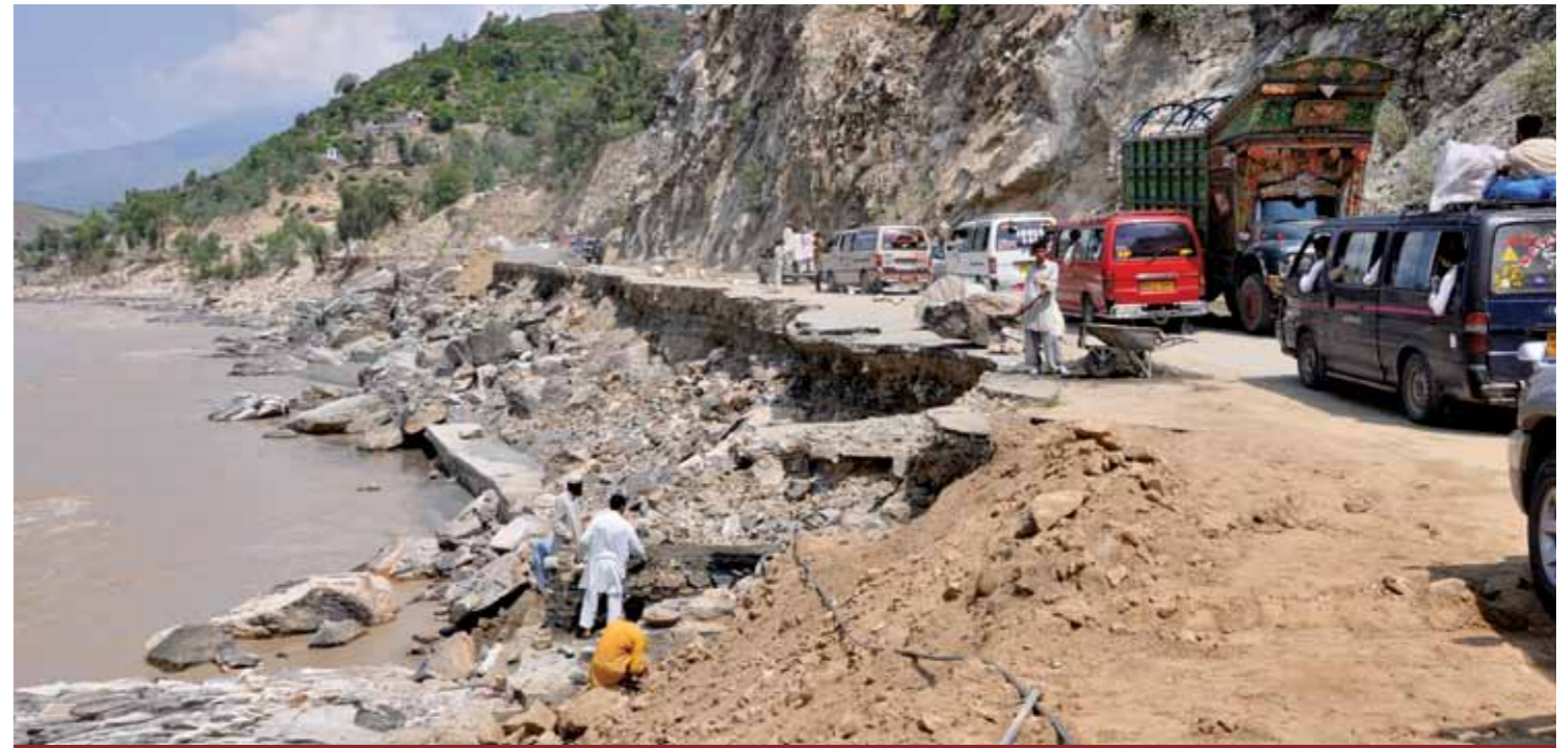
Floods washed away roads in Pakistan and made it difficult to bring urgent supplies to flood-affected areas. The rebuilding of roads is part of the long-term disaster recovery.
