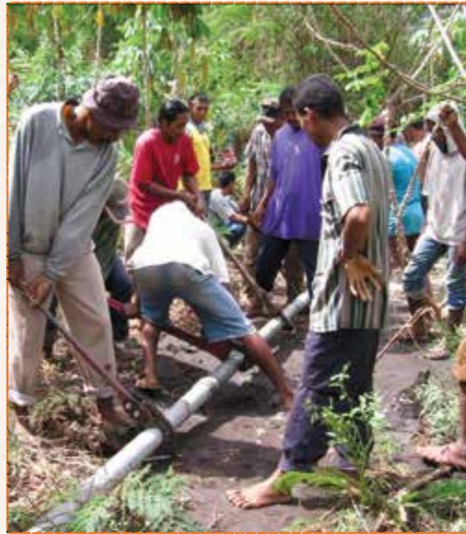
Every day, 50-60 men from the villages worked to build the pipeline. Construction took 16 months to complete.
