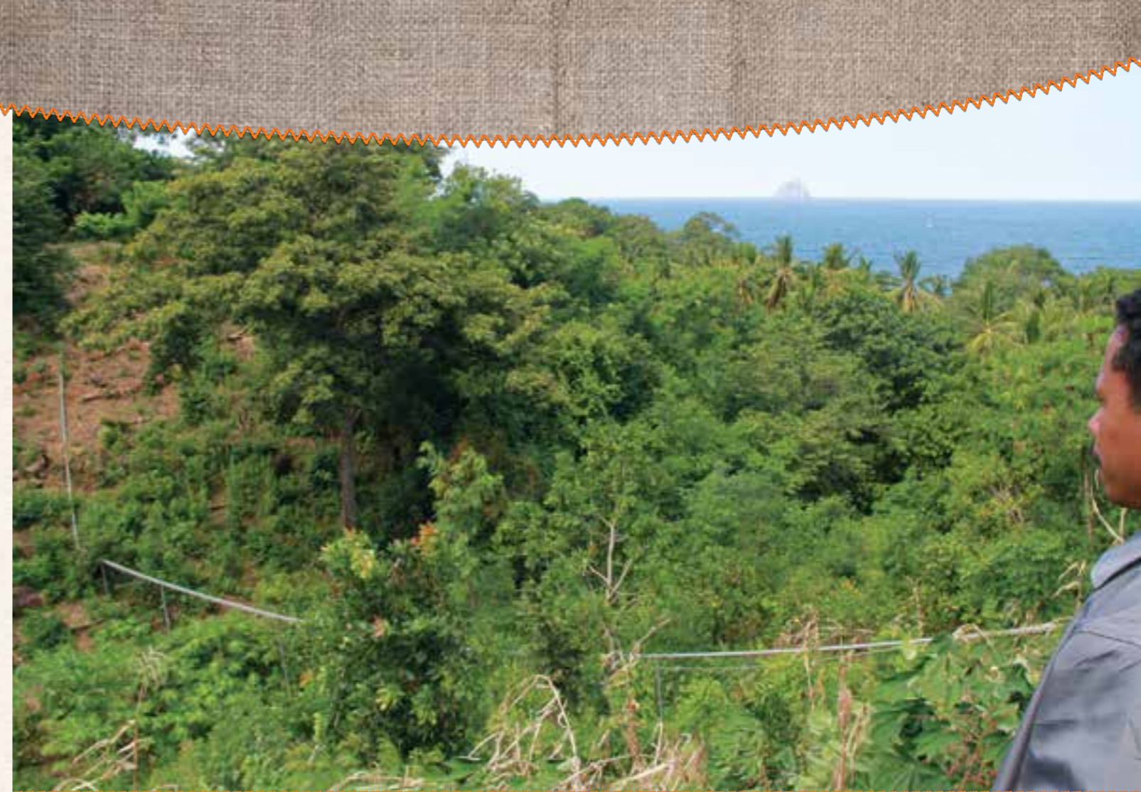
The gravity fed pipeline crosses valleys on its 27-kilometre trek from the water source to Kaha.
